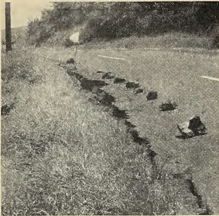
FIG. 9. Crack along roadside south of Kealakekua, from the south, showing separation of embankment from edge of pavement due to slumping.
